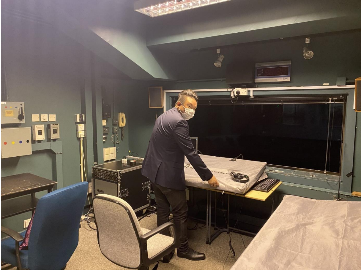
Control Room of the main Theatre
